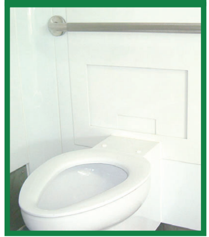
Toilet seat inside wash unit
